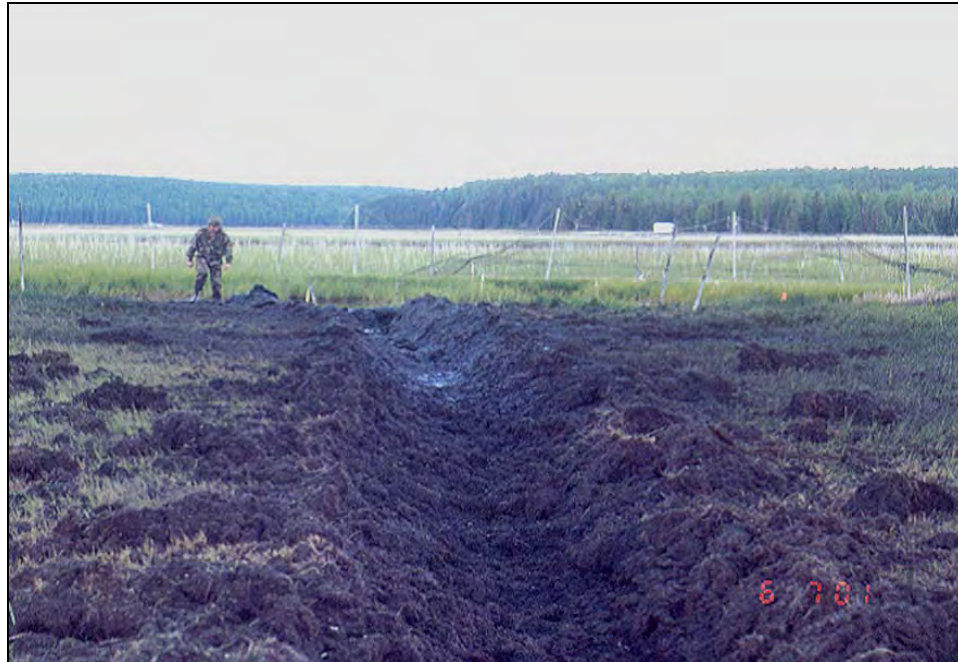
Figure 8. Drainage ditch at Pond 285 (Bangalores).
