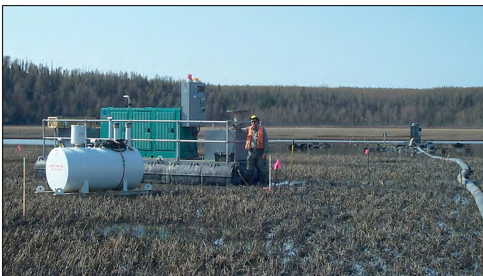
Figure 2. Pump system deployed at ERF.
